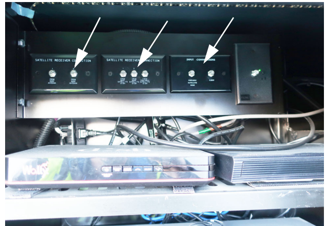
Satellite Dish Connections (Located in the passengers side front compartment door. -Typical View
