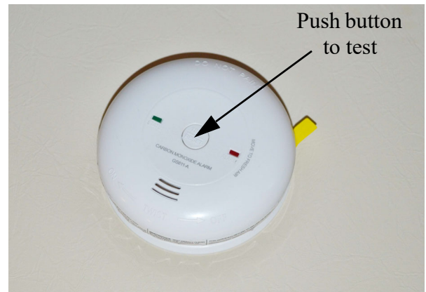
Carbon Monoxide Alarm
