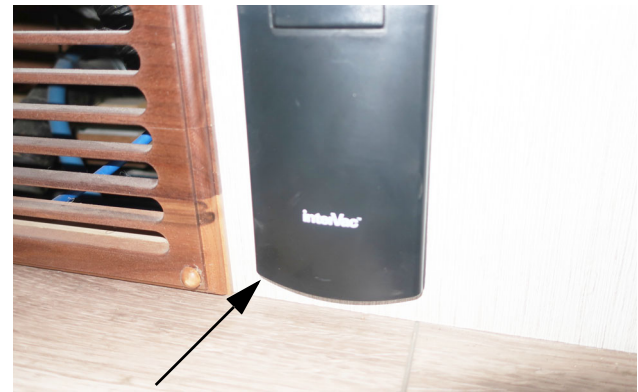
Interior Hose Outlet- lift cover to access -Typical View
