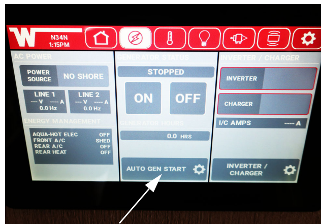
Generator Switch and Hourmeter (Located on multiplex monitor panel “Electrical” Screen) -Typical View
