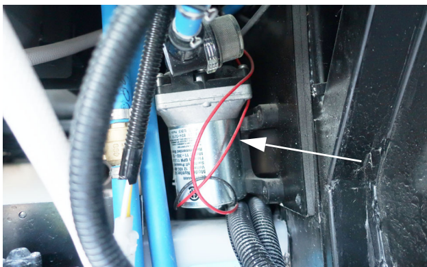
Water Pump (Located below the water center panel) -Typical installation shown
