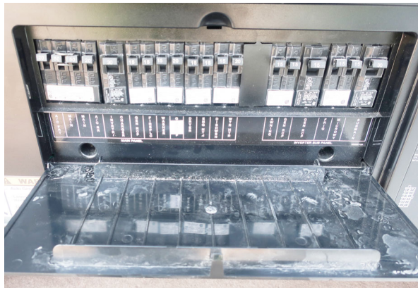
House Circuit Breakers -Typical Installation -Typical View
