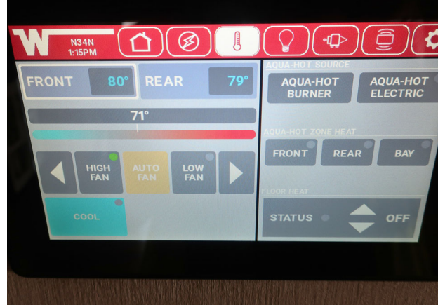
Hydronic Heating System Interior Control Switches "Climate" Screen -Typical View
