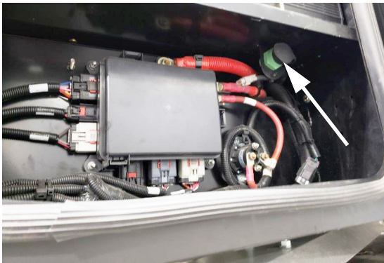
Diagnostic Plug (Located in the passenger side rear access compartment) -Typical View
