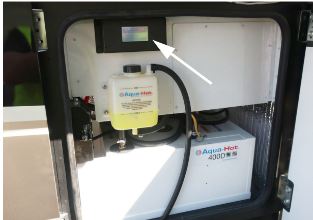
Monitor Panel located above the Expansion Fill Tank. -Typical View
