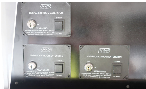
Slideout Switches (Located above entrance door) -Typical View
