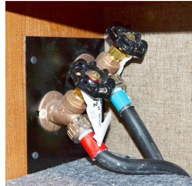
Water Supply Faucets -Typical View
