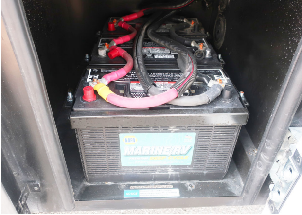
Chassis Batteries (Located behind a rear driver side exterior door) -Typical View
