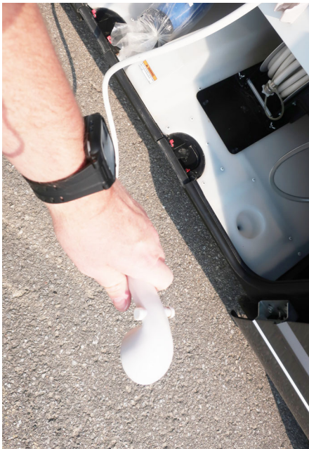
Using exterior shower to drain waterline -Typical View
