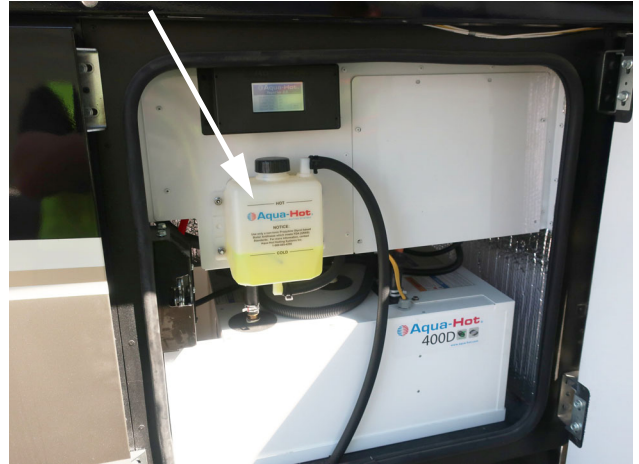
Hydronic Heating System (Located in passenger side compartment) -Typical View
