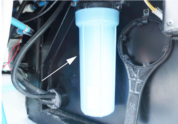
Waterline Drain Valves (Located in the water service center) Remove the filter to drain the water lines -Typical View
