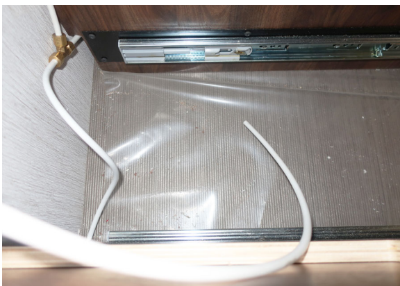
Inside the compartment is the drain line. -Typical View
