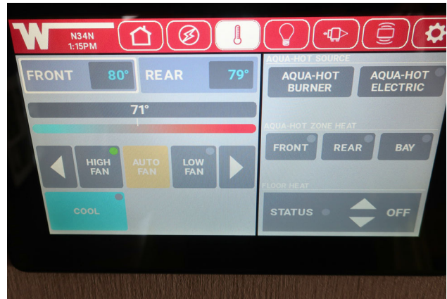
Thermostat "Climate" Screen (Located on Multiplex Monitor Panel)
