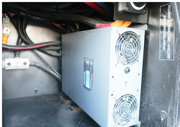
Inverter Charger Unit (Accessible through mid-passenger side compartment door) -Typical View
