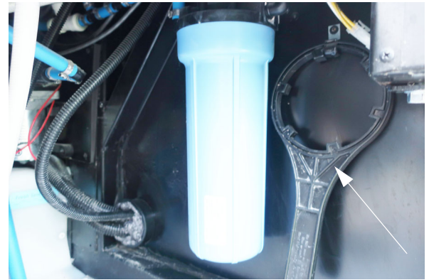
Filter Wrench (Located in water service center) -Typical View
