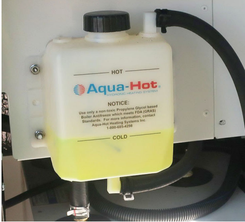
Expansion Fill Tank -Typical View
